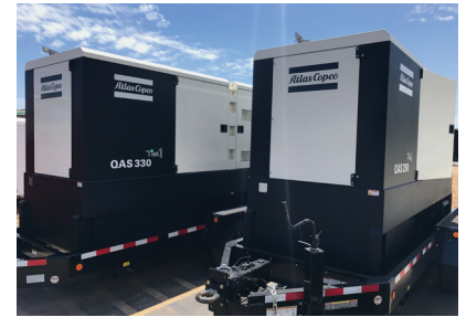
Portable & Standby Generators
